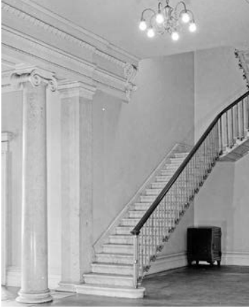
Carrara marble staircase, Beverwyck, Library of Congress, Historic American Buildings Survey/Historic American Engineering Record/Historic American Landscapes Survey
